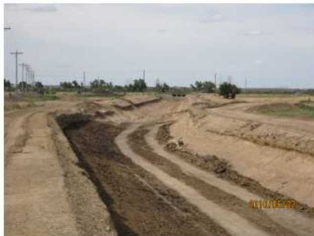
Clay liner being placed near Station 114+00, looking north towards the River Road bridge.
