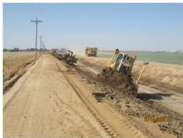
Grading and compacting of the cover layer north of the turnout/drop structure.
