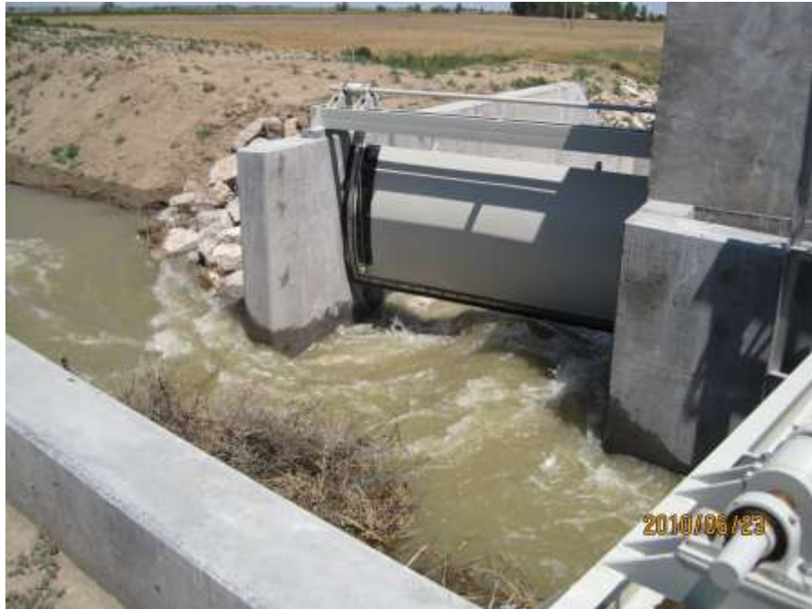
South Side ADS new bifurcation control structure. Back when there was river flow, Water can be seen flowing under the return gate headed back to the river.
